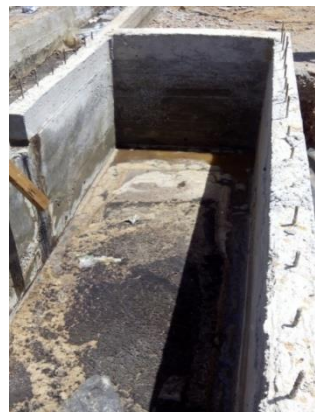
Figure 2. Photography of leachate collection basin
